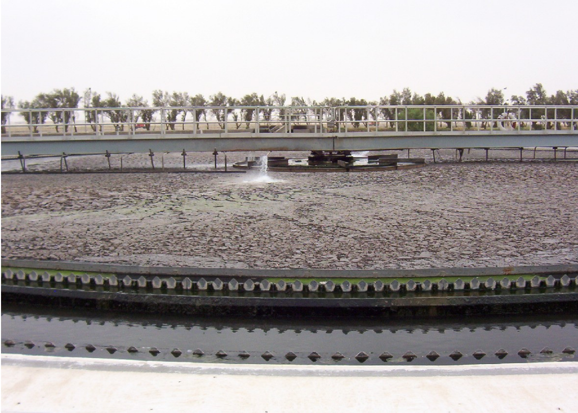
Fig. 2 Floating sludge in clarifier.
